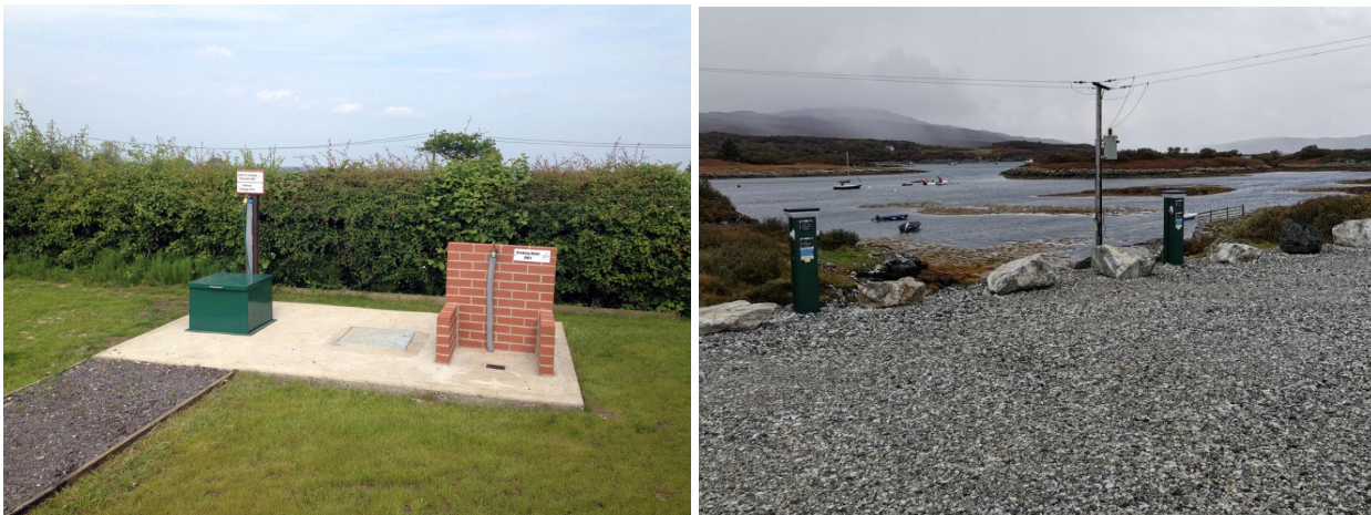
Figure 2. Left - example of water tap and Chemical Disposal Point, Right - electric hookup points at an aire in Mull.
